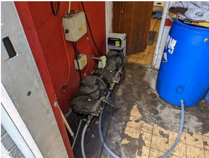
Figure 6: Pump for the pressure washer with electrical cables and hoses causing trip hazard, Leicester
