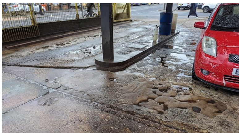
Figure 15: Wash pad with severe corrosion due to use of cleaning chemicals including acid. Leicester
