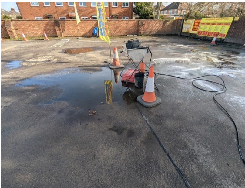
Figure 11: Pooling at a hand car wash, the surface is not designed to handle capacity. Suffolk
