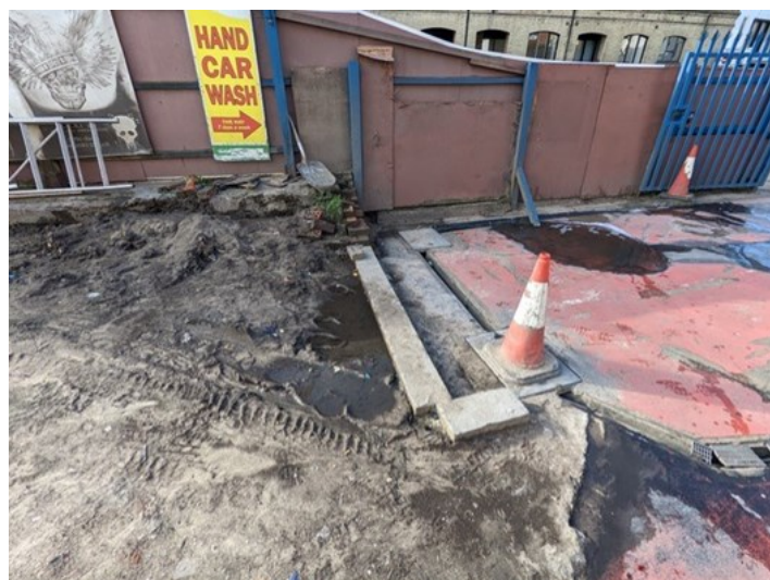
Figure 5: Uneven terrain, broken drain covers and large pools of water. Suffolk
