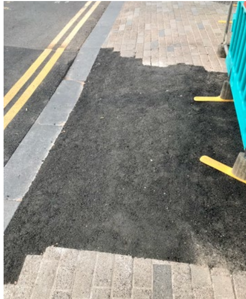
A recently laid, and more recently ruined pavement, in Stoke-on-Trent
