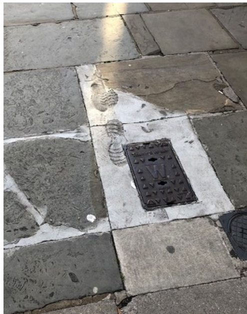
Cleveland Street, West London. Is concrete an appropriate replacement for York Stone? This scar is at least two years' old.
